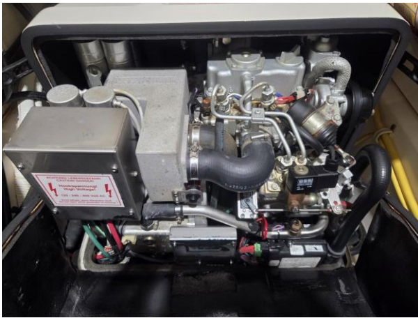
36 Generator well mounted; motor mounts secure and clean.
