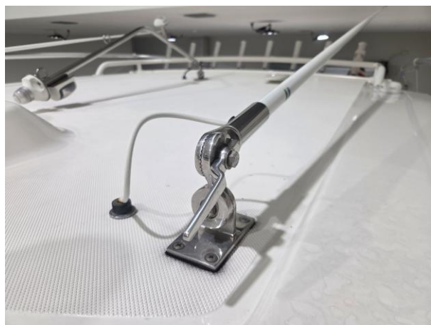
67 DEF-15: VHF antenna coax exposed at the base with no UV protection.
