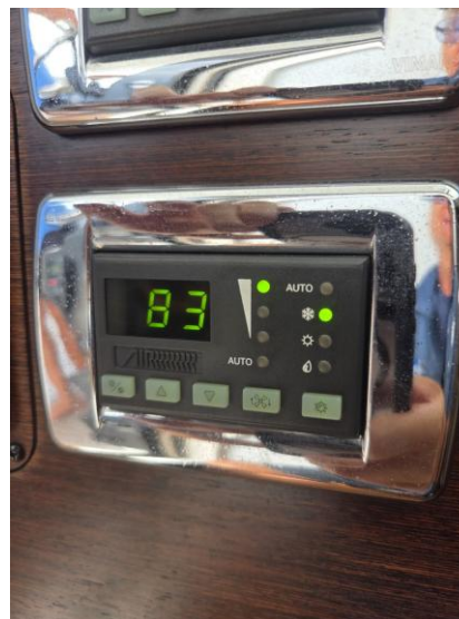
64 DEF-9: Upper-deck (No. 2) air-conditioning control read approximately 83 degrees F; unit did not produce cold air.
