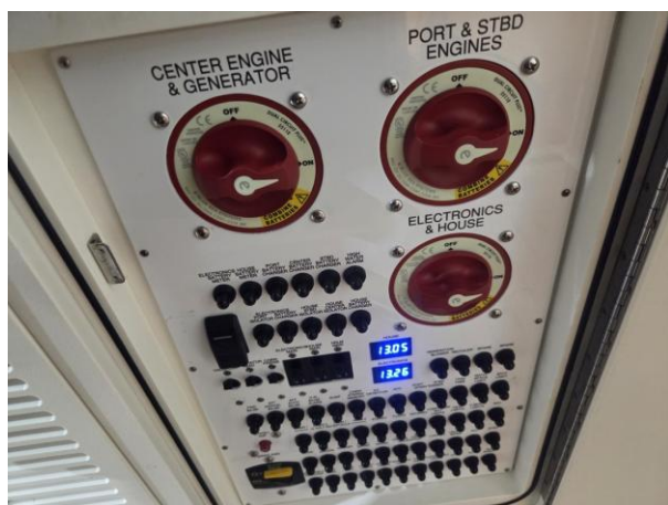
22 Battery switches readily accessible on the main DC panel beneath the helm seats.
