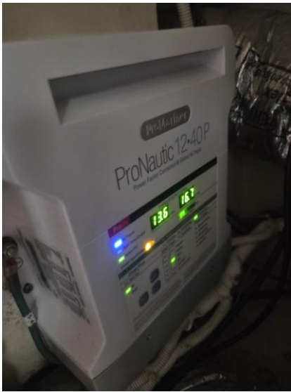
26 Bow-thruster battery charger.
