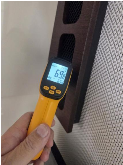
50 Cabin (No. 1) air-conditioning output measured 69 degrees F.
