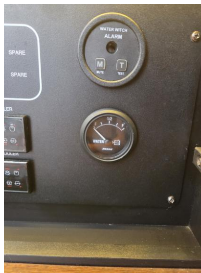
41 Bilge high-water alarm tested.
