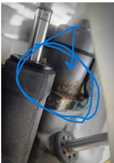
61 DEF-6: Trim/tilt motor case corrosion, typical of all three engines.
