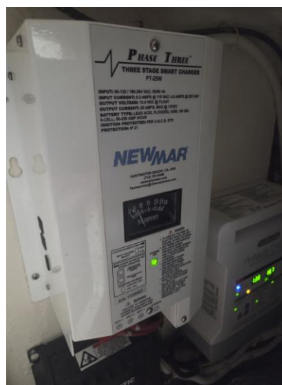
25 House-battery smart charger.
