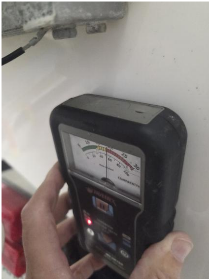
57 DEF-1: Elevated moisture-meter reading (Tramex Skipper) at the transom, engine-mount area.
