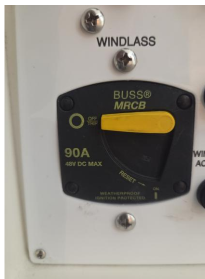
23 Main DC breaker on the main DC panel.
