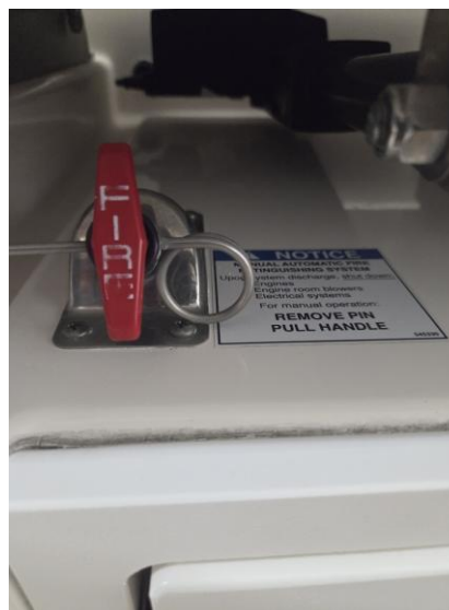
43 Fixed fire-suppression manual activation readily accessible at the helm.
