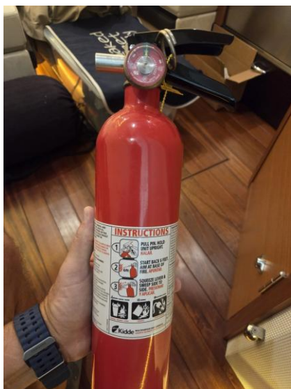
42 Three hand-held fire extinguishers, all current.
