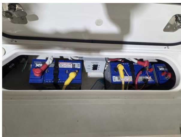
24 Batteries well secured and protected, insulated terminals per ABYC E-10.
