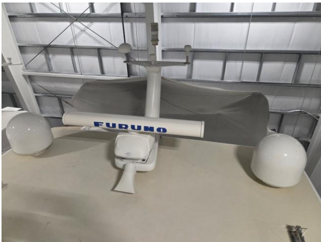
49 Furuno open-array radar powers up
