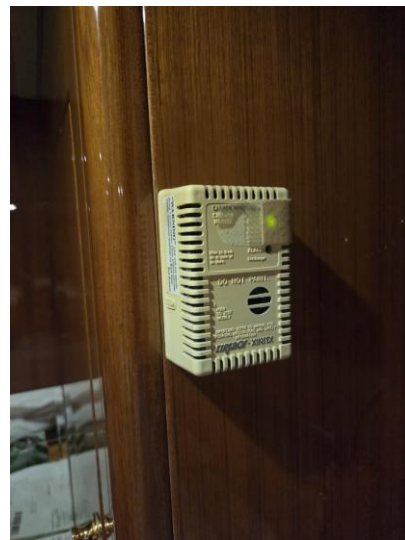
88 CO / smoke alarms show green readiness indicators
