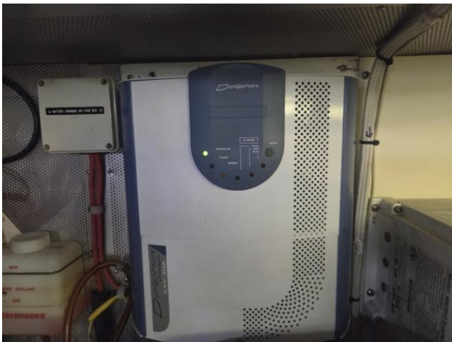
39 Dolphin marine battery charger
