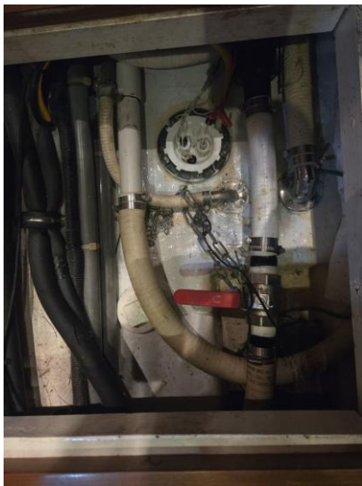
71 Holding tank well secured
