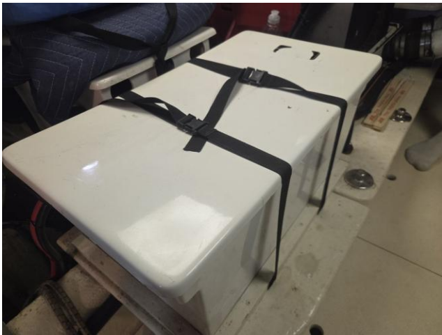
37 Batteries in ABYC-approved marine-grade battery boxes
