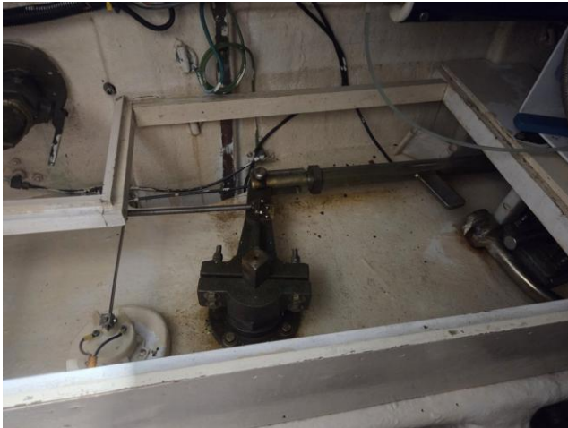
33 Steering gear in a protected compartment — clean, lubricated and adjusted
