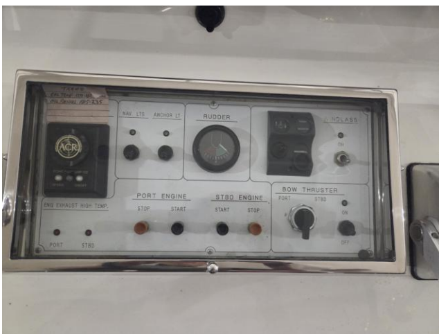
55 Flybridge searchlight, rudder indicator and bow thruster controls — enclosed and protected from weather
