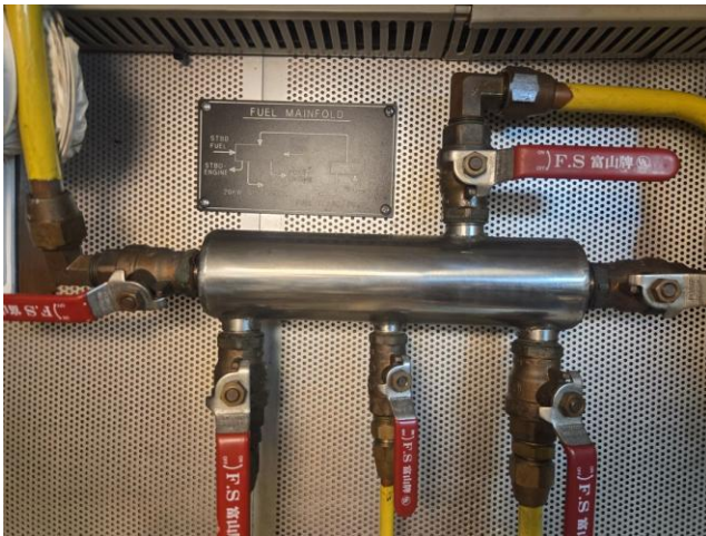
63 Fuel control manifold well labeled
