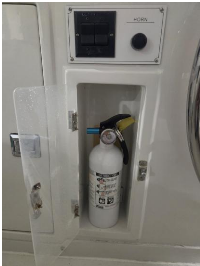
83 Handheld fire extinguishers readily accessible
