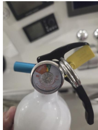
84 Extinguisher gauge in the green
