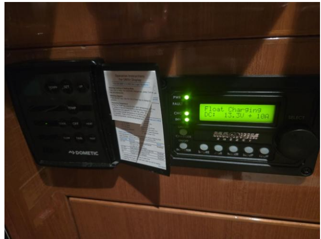
38 Battery management — float charging 13.3 V, appears accurate
