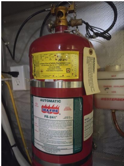
81 Sea-Fire FE-241 fixed fire suppression — serviced 12/30/2025
