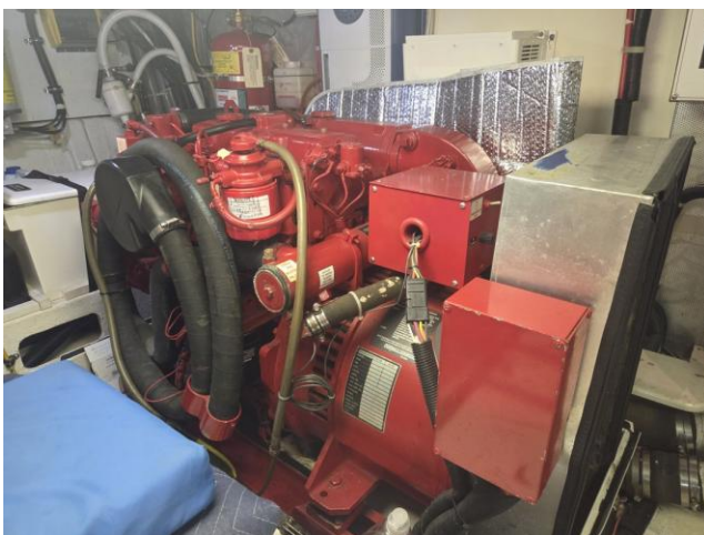
41 Westerbeke 20 kW generator
