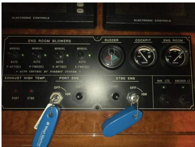
29 Engine room blowers — all power up; manual/auto control from the pilothouse
