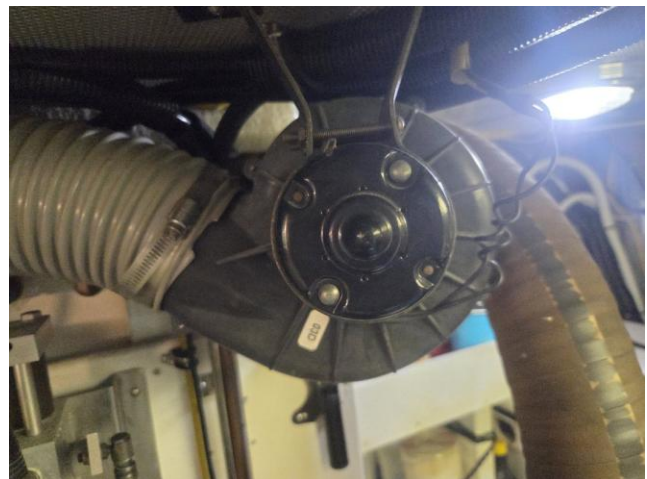
30 Engine space forced-air ventilation blower powers up
