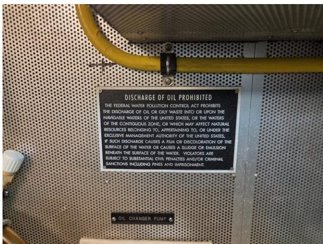
89 USCG "Discharge of Oil Prohibited" placard sighted
