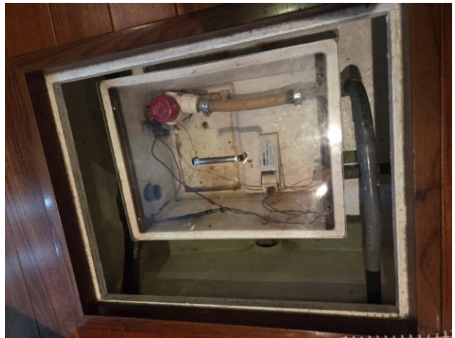
70 Grey-water sumps clean and operational
