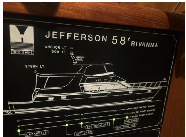
90 Jefferson 58' Rivanna systems status panel
