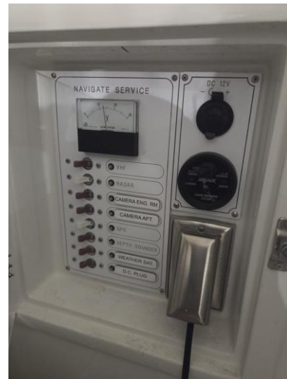
40 Flybridge DC panel well protected
