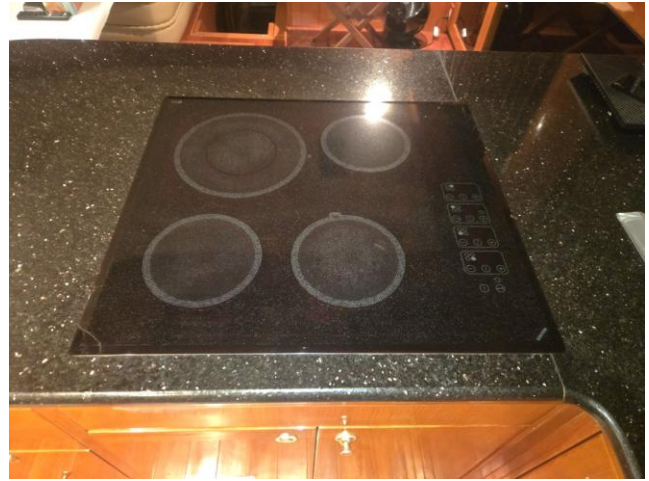
92 Galley four-burner electric glass cooktop
