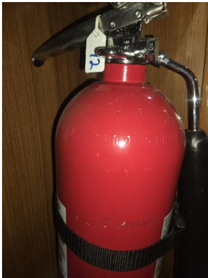
85 5 lb CO2 extinguisher secured in bracket
