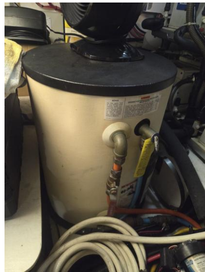
72 Water heater pressure relief properly plumbed to the bilge
