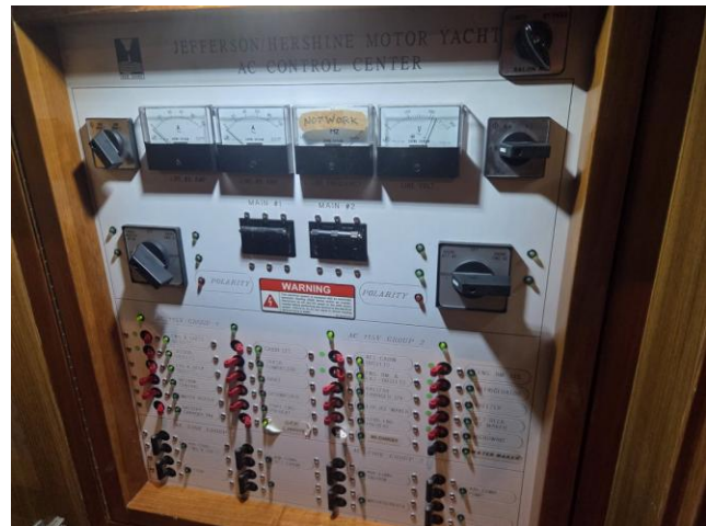
36 Main AC control center with metering
