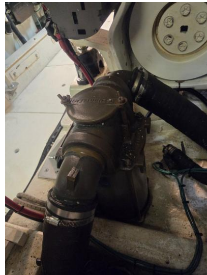
26 Main engine raw-water strainers clean, corrosion-free and well bonded; hoses and clamps serviceable
