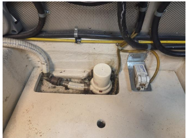
66 All bilge pumps and high-water alarms operated with no exceptions
