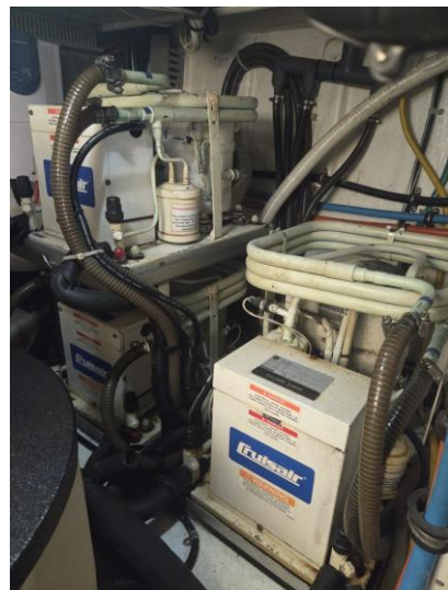
74 Cruisair air-conditioning units
