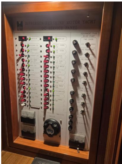
35 Main DC distribution panel
