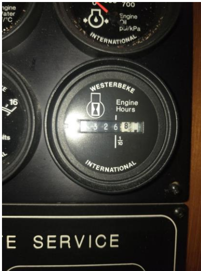
43 Generator hour meter — 1,326 hours
