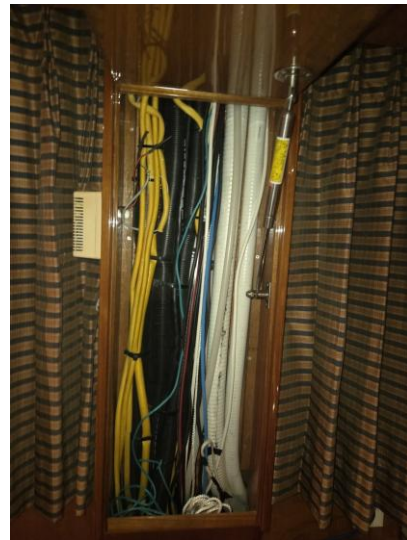
44 Wiring chases neatly dressed and supported
