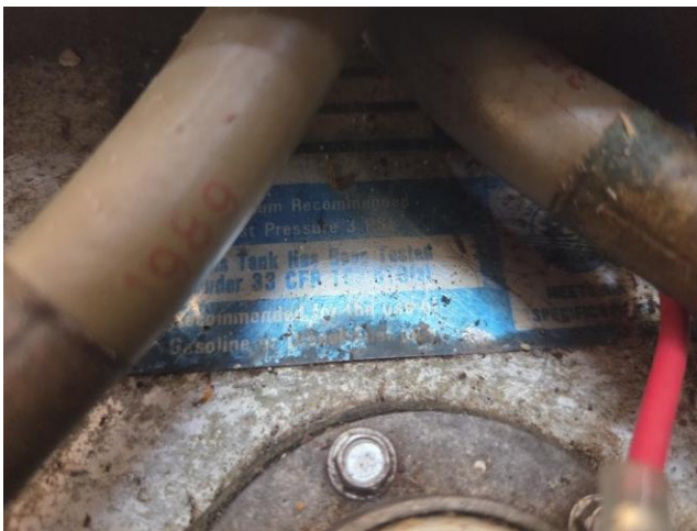
57 Fuel tank identification label present, not completely legible
