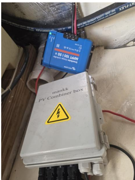
49 DEF Victron charge controller and PV combiner box not mounted, adrift
