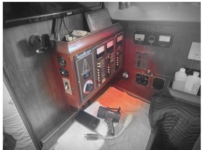
17 Chart table and main electrical panel
