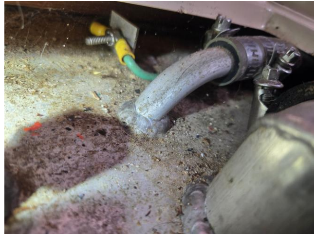
56 Fuel tank bonding terminal connection well established
