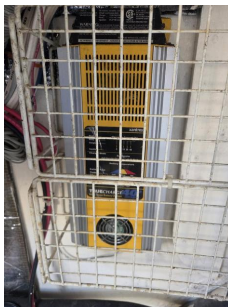
44 DEF 120 VAC battery charger does not power up
