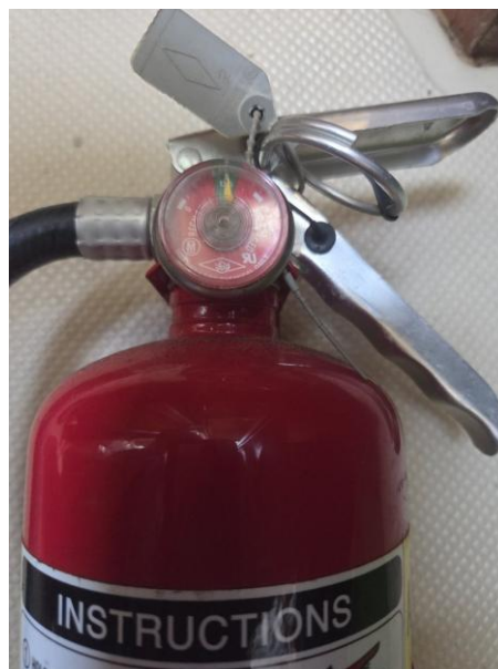
68 DEF All hand-held fire extinguishers are expired
