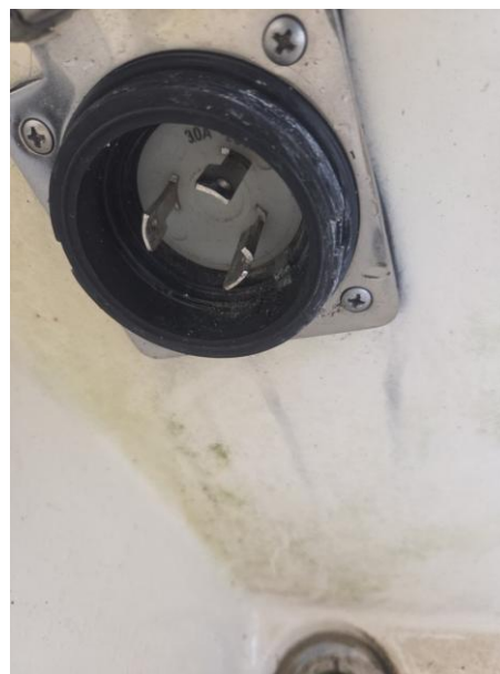
40 Shore-power inlet corrosion-free; no evidence of high heat or resistance
