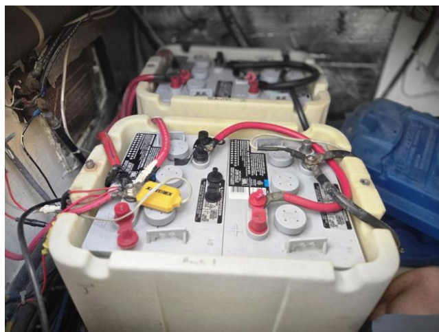
41 Batteries in marine-grade, non-conductive boxes with protective covers, per ABYC
