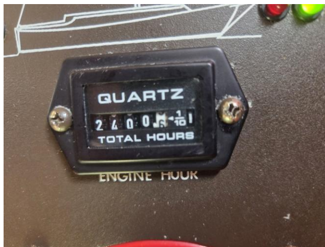
25 Panel engine hour meter — 2,400.6 hours
