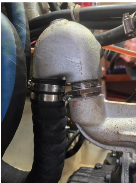
28 Engine exhaust well secured and leak-free
