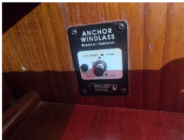
50 DEF Anchor windlass breaker; windlass removed and power cables adrift in the chain locker
