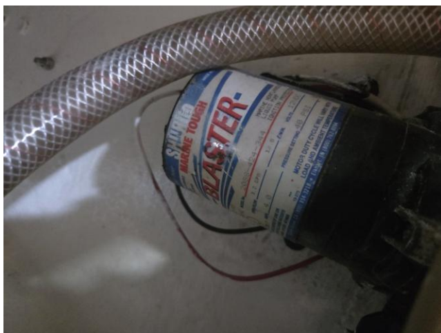
61 DEF Raw-water washdown pump inoperative
