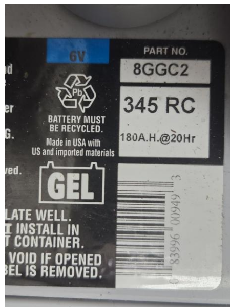
42 6-volt GEL battery, 180 Ah — two in series in each enclosure
