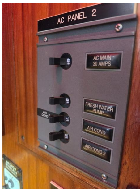
39 AC panel 2 — all circuits well marked
