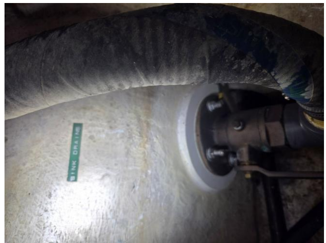
58 Seacocks operate open and closed — sink drain seacock shown
