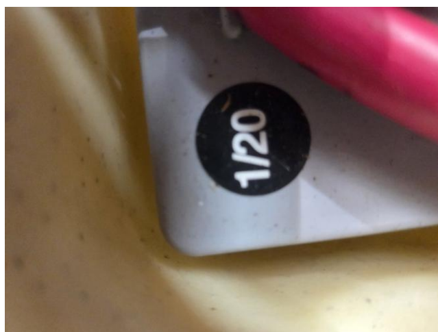
43 DEF Batteries date-coded 1/2020 require replacement
