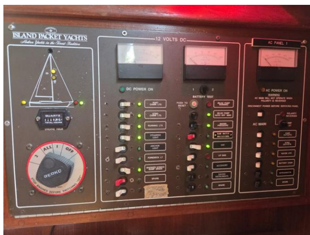
37 Main electrical panel; battery switch readily accessible
